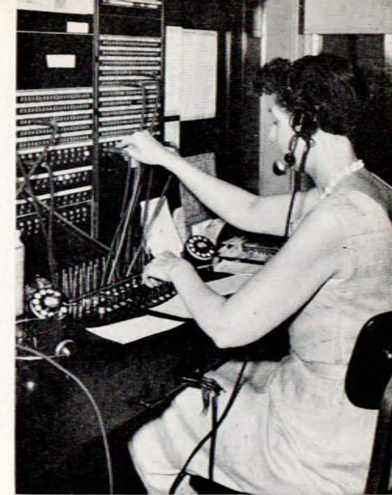
There are 400 locals, 37 trunk lines to contend with . . . .
