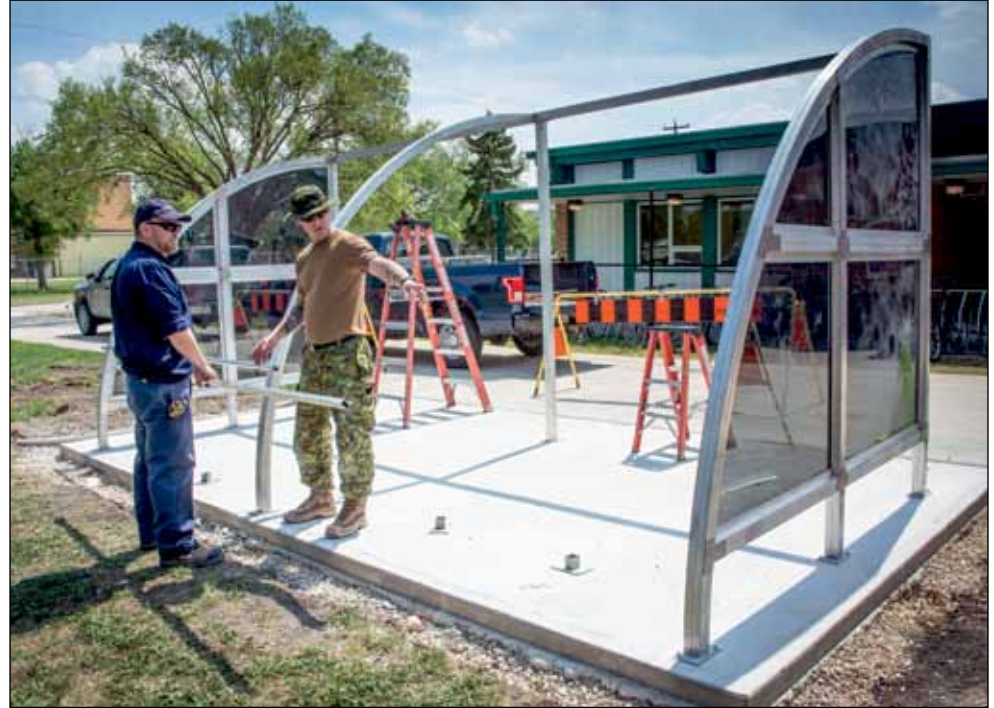
George Duncan, RP Ops, and Cpl William Reimer, Wing CE Flight, set up a new bike shelter in front of Building 90 on May 23, just in time for the RCAF Run. Photo: Bill McLeod, Voxair Manager
