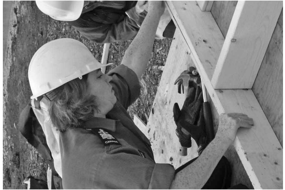
HMCS Winnipeg Cox'n CPO1 Janet Graham-Smith helps build the framing for one of the Habitat for Humanity homes under construction in Winnipeg. Photo: Gloria Kelly, NDPAO
